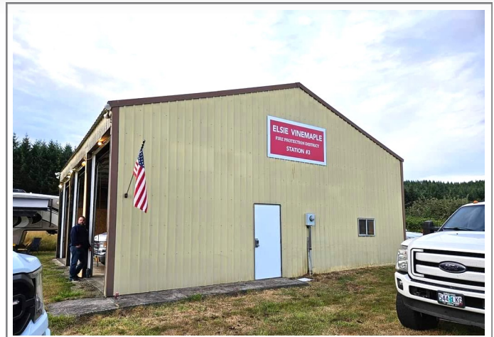
Volunteers, wearing masks and gloves, tore out all the rotted and destroyed portions of the inside, hauled away numerous truckloads of debris, scrubbed it inside and out, painted the door, and added a new sign and a flag.
